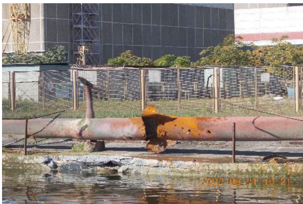
Broken pipe observed by ISAMZ at the ZNPP site due to shelling on 21 September (Photo: IAEA)
