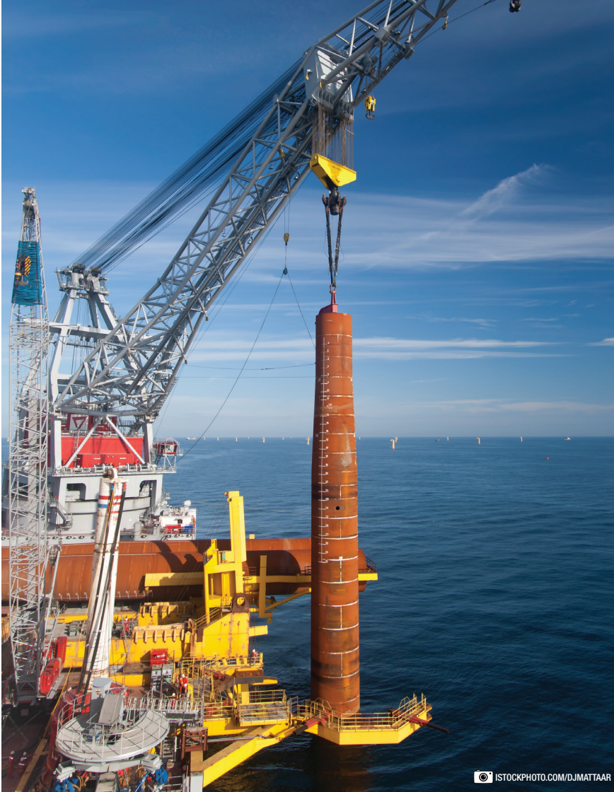
Figure 4: Pile driving is used for the construction of offshore windfarms, piers, and bridges, for example. Pile driving noise abatement systems could reduce sound exposure levels using a combination of systems.
